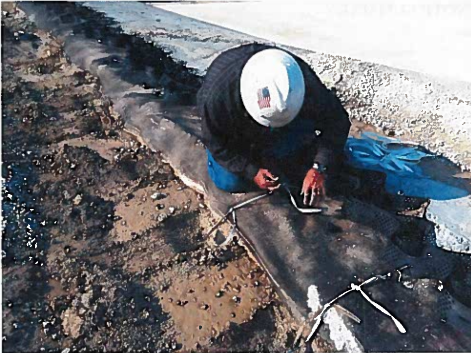
Brieser repairing cut geocell tendons along the pond access road (looking southwest).
