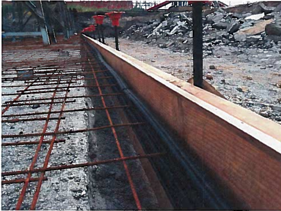
HDPE embedment strip installed on forms in preparation for concrete placement (looking east).
