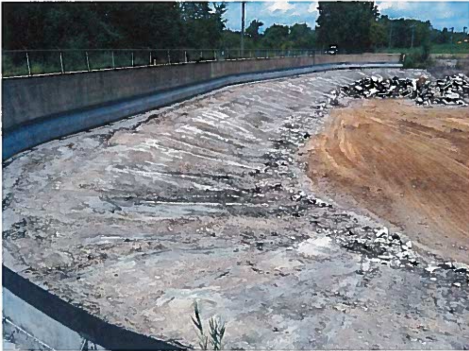
West slope prior to grading the soil near the weir (looking north).
