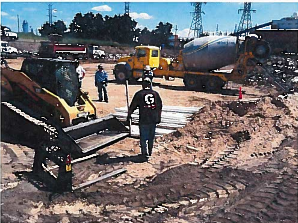
PVC pipe being filled with sand for use as the geocell deadman in the anchor trench (looking northeast).
