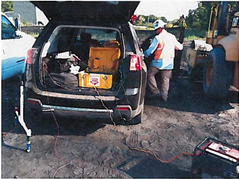
Liner integrity survey power supply and other equipment (looking north).
