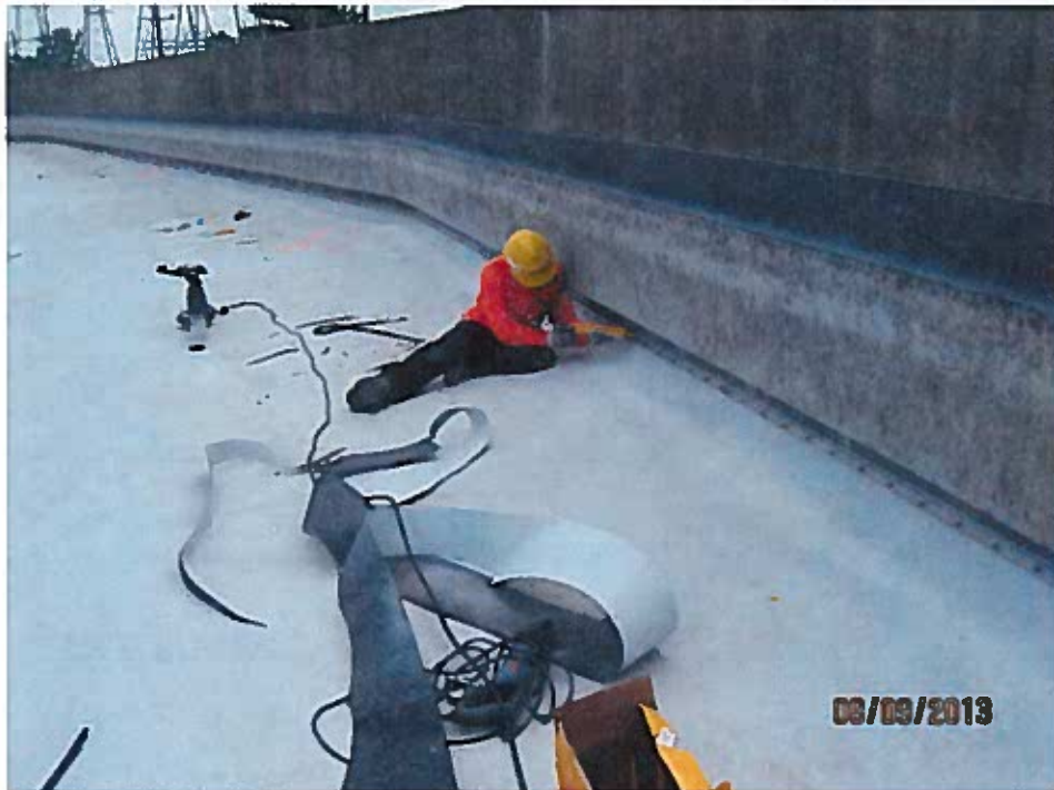
Calking geomembrane termination above the batten strip along the weir wall (looking southwest).
