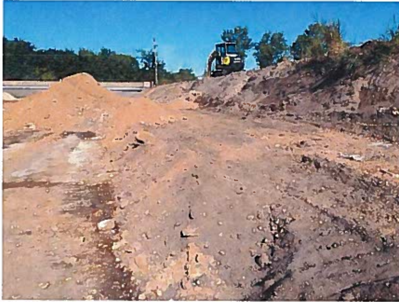
View of improperly placed material for slope reconstruction, facing west
