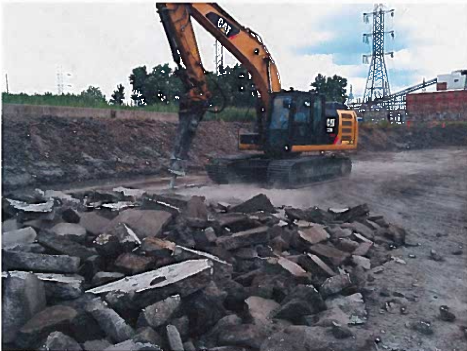
Excavator with hammer breaking up the Poz-o-Pac in the pond (looking northeast).
