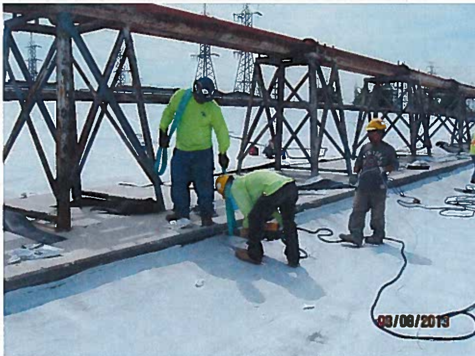
Extrusion welding geomembrane to HDPE embedment strip in the concrete pad (looking southwest).
