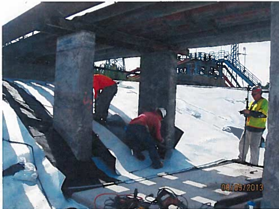
Installing geomembrane below pipes on east slope. Surveyor documenting panel seams and repair locations (looking southeast).
